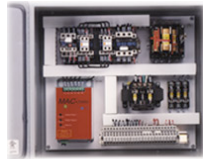
Mac•2000 Control Panel
